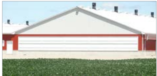
Figure 1. Tunnel ventilation inlet doors across the end wall of a barn without evaporative cooling.
