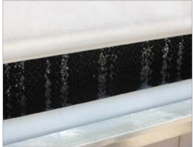
Figure 8. Close-up of water trickling down the outside of the pad surface.
