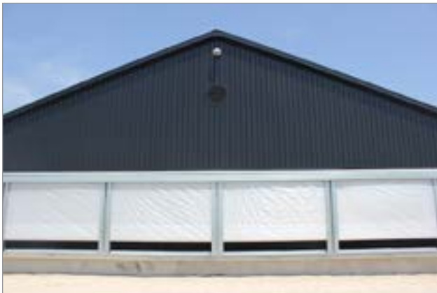
Figure 11. Evaporative cooling pads with protective covers (white tarp material) partially closed.
