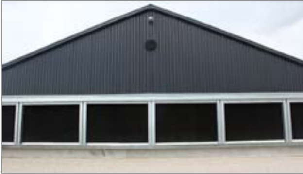
Figure 3. Tunnel ventilation inlet with evaporative cooling pads installed.
