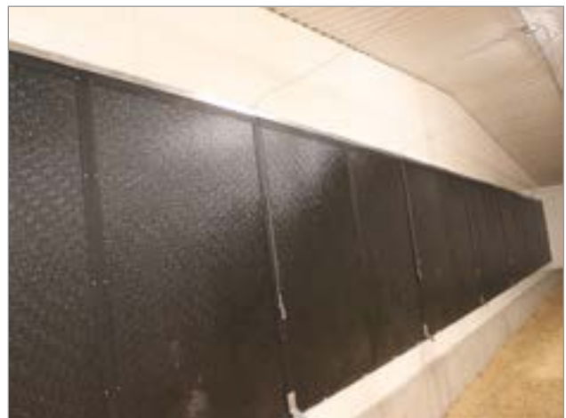
Figure 10. Insulated door closed to cover the evaporative cooling pad.
